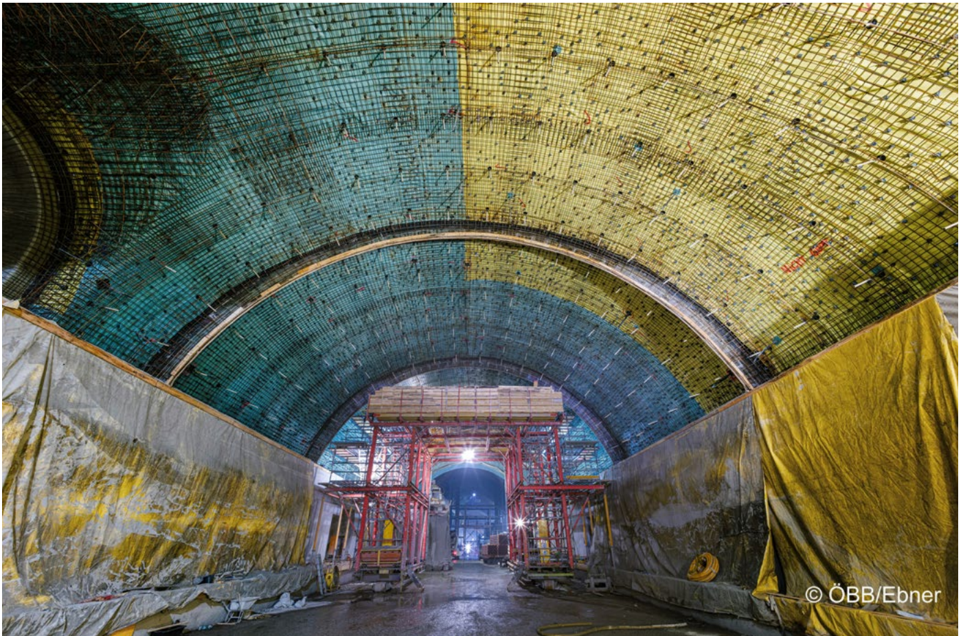
Emergency stop, Semmering Base Tunnel, Austria
